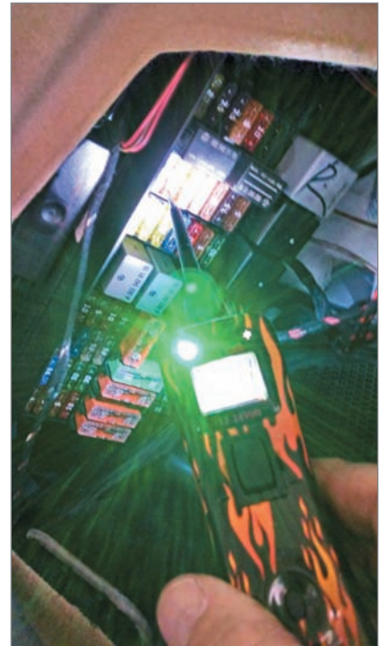
Power Probe shows ground on Circuit 15
