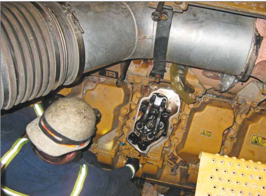
(Left) Ultra cleanliness and exact torque procedures need to be top priorities when changing injectors in a C175.
