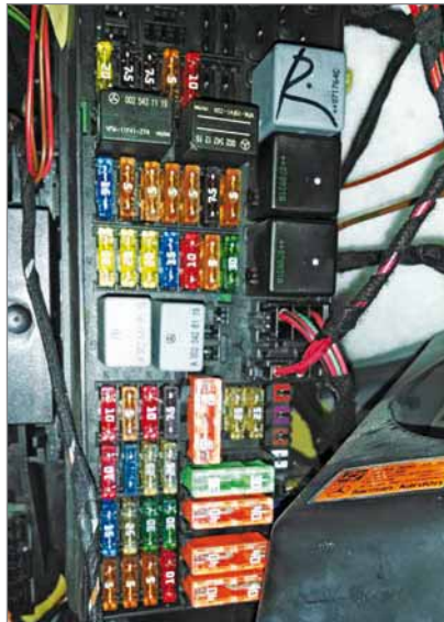
Lots of places for problems in a fuse box.
