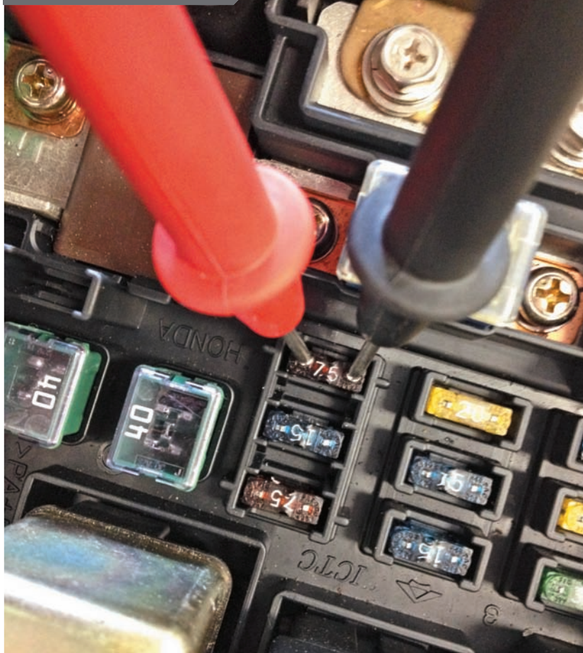
Voltage drop testing across a fuse is the author's preferred method for finding parasitic draw concerns.
