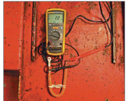
Here we're testing the cable and making sure it's not shorted to the shielding. Meter reading is 2.2 Gigohms.
