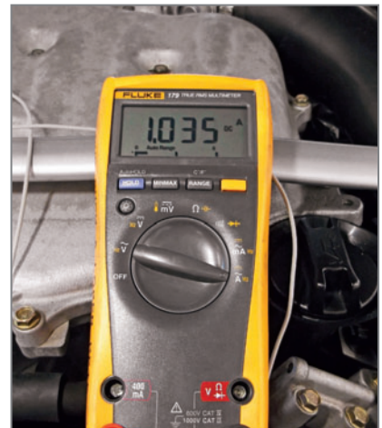
Using an amp meter and jumper leads, we checked amperage draw of AF sensor 1's heater circuit at the sensors harness connector.
