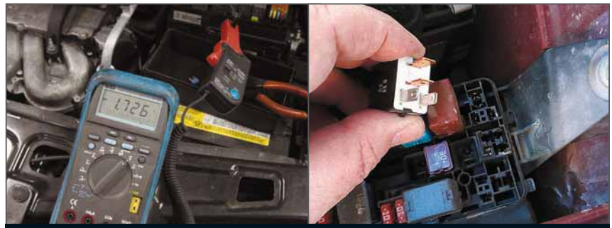
(Left) You can quickly determine which of the two circuits needs your attention using a low amp current probe and your meter. (Right) The relay lies in the intersection of the circuits it is a part off and needs to be considered as a load AND a control.
