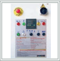
Electromechanical control panel.
