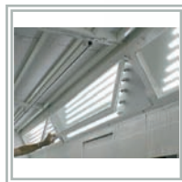
Eight 6-Tube light fixtures with hinged access for ease of cleaning and maintenance.
