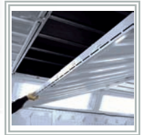
Hinged ceiling filter frames for easy replacement of 10 micron media filters.
