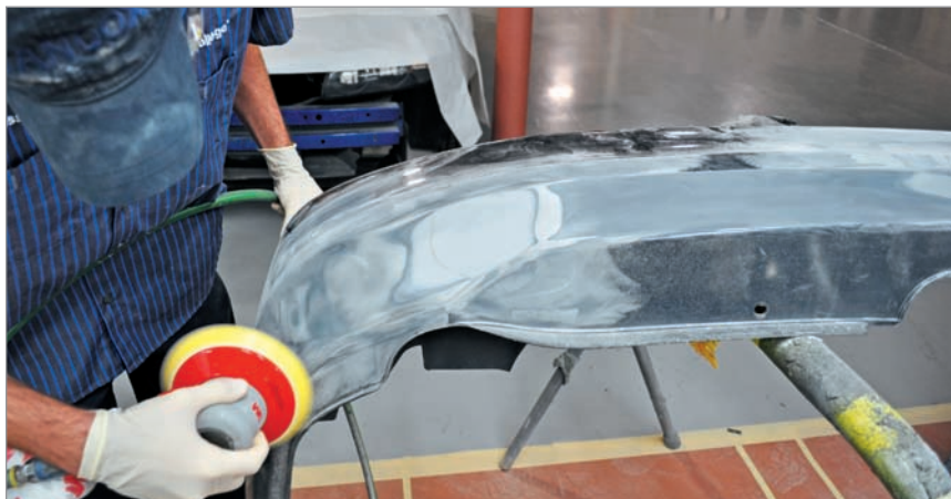
Adhesives require extensive sanding of the repair area to build the bond.
