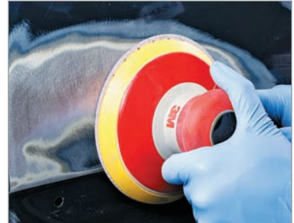
Using 80 grit sandpaper, remove all paint in a 2 in. area surrounding the repair.
