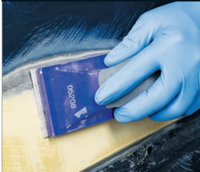
Use 180 grit sandpaper to level off the repair area and remove any of the 80 grit scratches.
