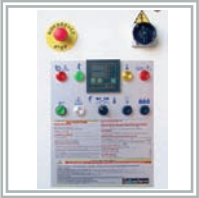
Electromechanical control panel.
