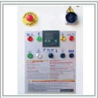
Electromechanical control panel.
